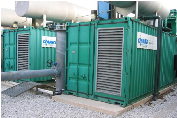
Clarke Energy Jenbacher gas generators installed at Brombrough Dock landfill site, Liverpool.
